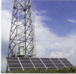
01 Signal transferring station
