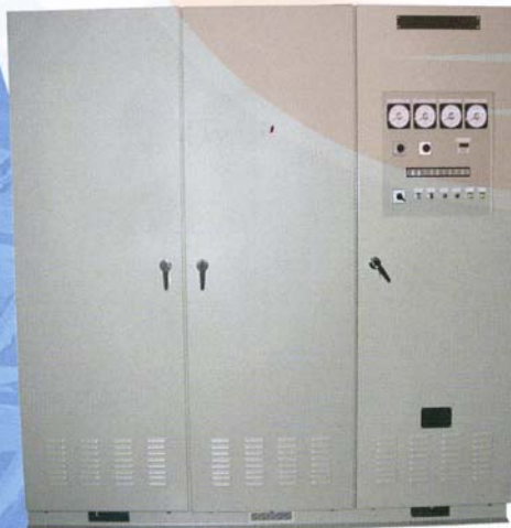
Air Cooled Rectifier for Hypochlorination
