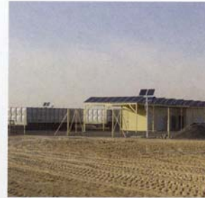
03 43 kWp Solar powered water pumping and desalination system (43kWp in Dubai, UAE)
