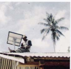
09 Remote solar home systems (50 kWp in Indonesia)
